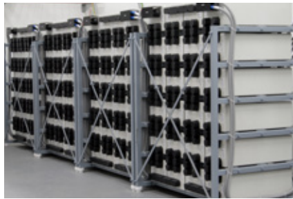
Energy Storage System
